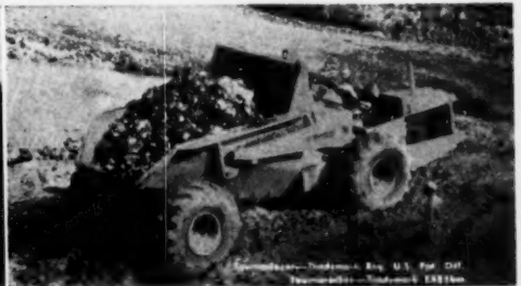
Mining bauxite at Onverdacht, Surinam, deep in tropical jungles, Billiton Mines of Paramaribo stripped 20 ft. of heavy, wet clay overburden with 3 C Tournarockers—liked them so well they bought 6 more for hauling ore.
